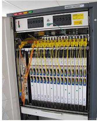
Gambar 3.4 OLT (Optical Line Terminal)
