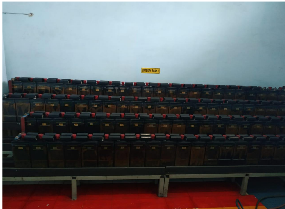
Gambar 2.9 Baterai Bank 1 110 V GI mabar (Sumber :Gardu induk Mabar,2019)
