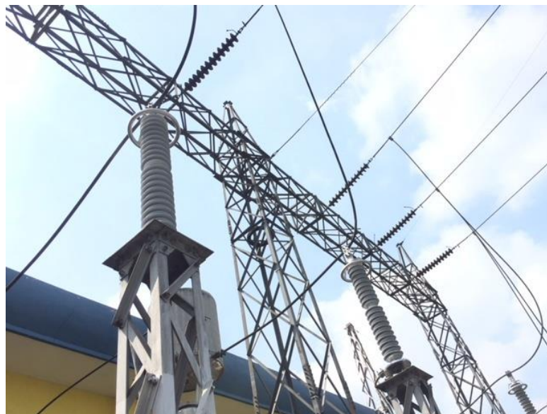
Gambar 2.7 Lightning Arester GI Mabar (Sumber :Gardu induk mabar,2019)
